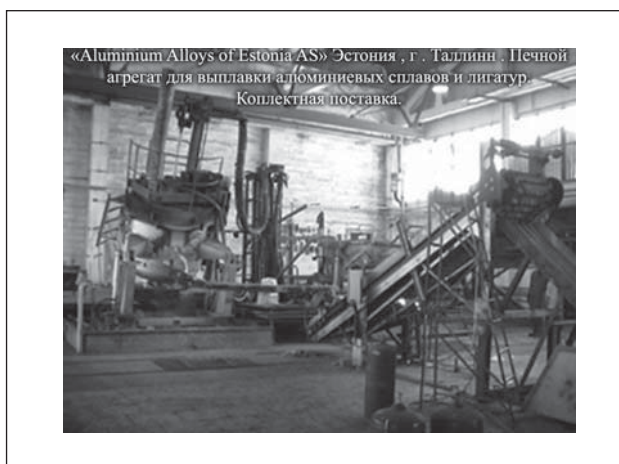
Fig. 9. Furnace for melting of aluminum alloys and alloying compositions at "Aluminium Alloys of Estonia AS" (Tallinn, Estonia). Full set supply
