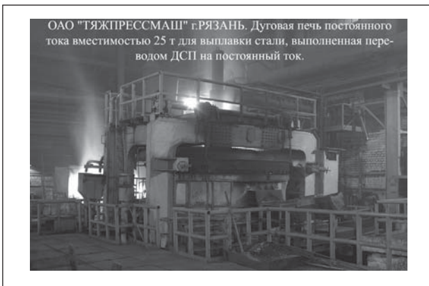
Fig. 2. GPDCAF-20 (JSC “Tyazhprommash”, Ryazan): 25 t capacity direct current arc furnace for steel melting made by switching ACAF into direct current
