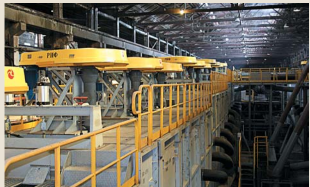
Reconstruction of flotation section of concentration factory "Almalyksky GMK" JSC, Almalyk, Uzbekistan
