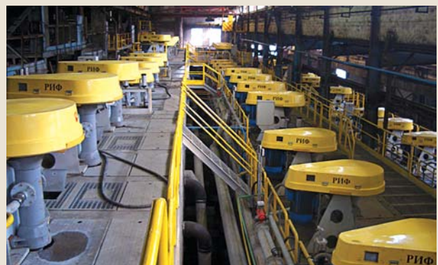
Reconstruction of flotation section of Concentration Factory of Zangezursky MMK, Kadjaran, Armenia
