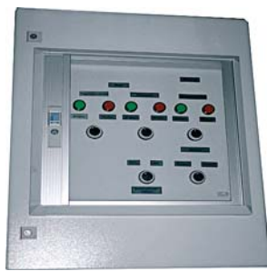
Fig. 5. Pneumatic box of control ShP-ZA with the elements of control and indication
