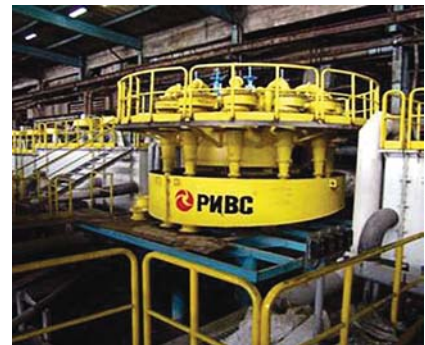
Fig. 3. Automated pump-hydro-cyclone unit involving twelve hydro-cyclones NPO "RIVS"
