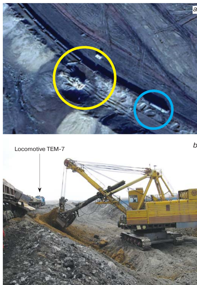
Fig. 1. Operation of shovel EKG-10 in internal dumping: (a) satellite image; (b) land photography
