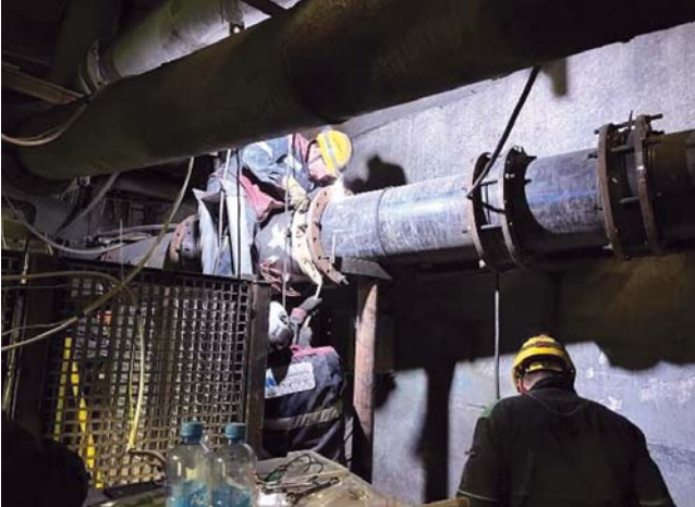
Fig. 7. MPP supervision installation (photo by authors)
