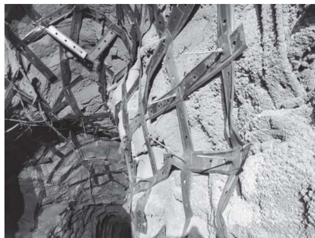
Fig. 2. Corrosion of metal strips, Severny site, Kupol mine, level +400 m (5 December 2019 photo courtesy I. S. Romanov)
